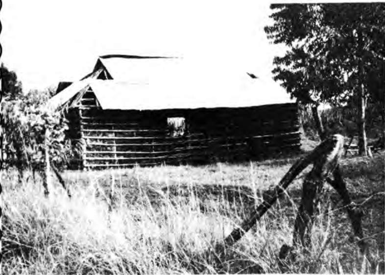
A new church building. The church didn't have the money to complete the roof.
